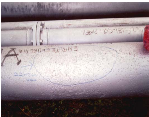
Figure 2 - Pitting on the surface of the 10 inches diameter pipeline.
