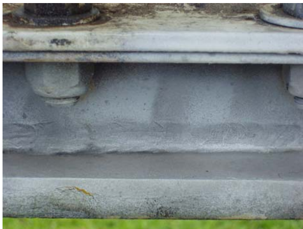
Figure 5 – Photograph white contrast paint being applied on fillet weld of the truck turntable.
