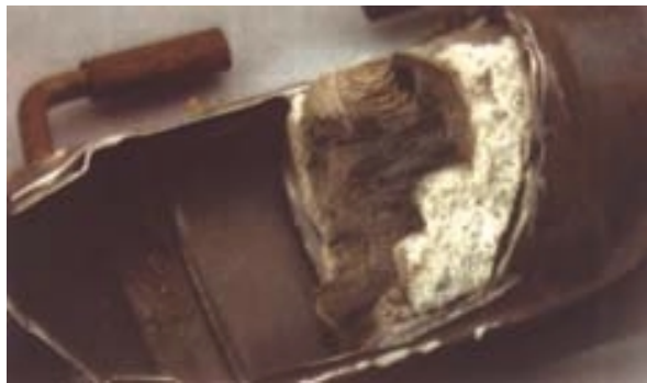
Fig-4a. Melting of CC due to overheat
