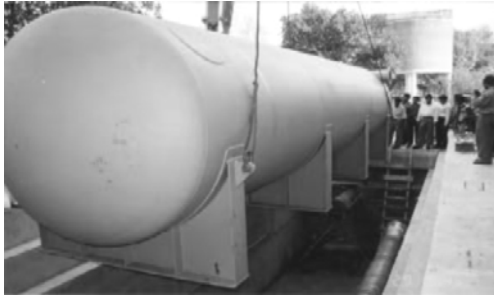
Fig 4: New decay tank with aluminium saddle
