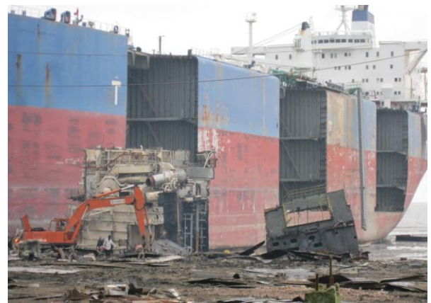
Fig 3. Hazardous working environment in ship breaking
