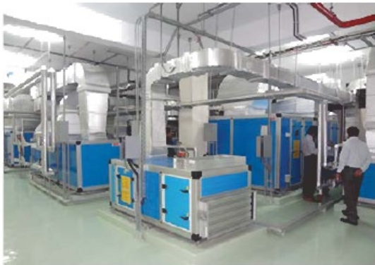
Inspection of HVAC System
