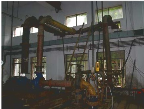
Pump Test Bed
